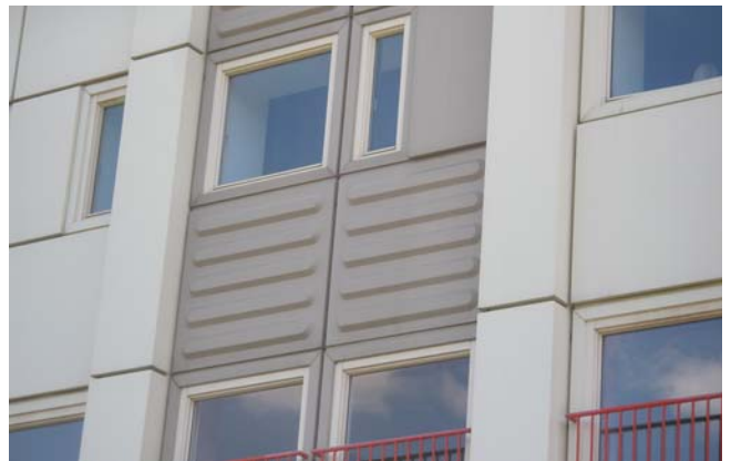
Hyde Park, Sheffield, remains pristine after 25 years and meets today's U value standards.
